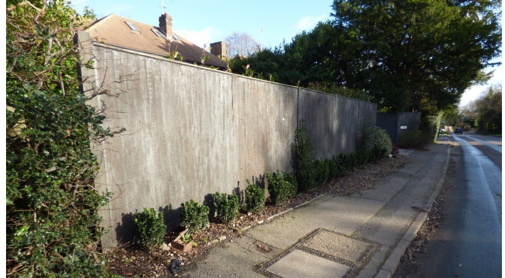
Figure 60: The removal of planting has had a suburbanising impact on some parts of the Conservation Area. In time the new planting will obscure the fence.
